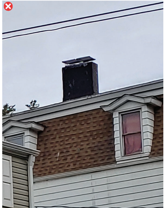
Incompatible metal chimney cap replacement; chimneys should have clay, slate, brick or stone caps
