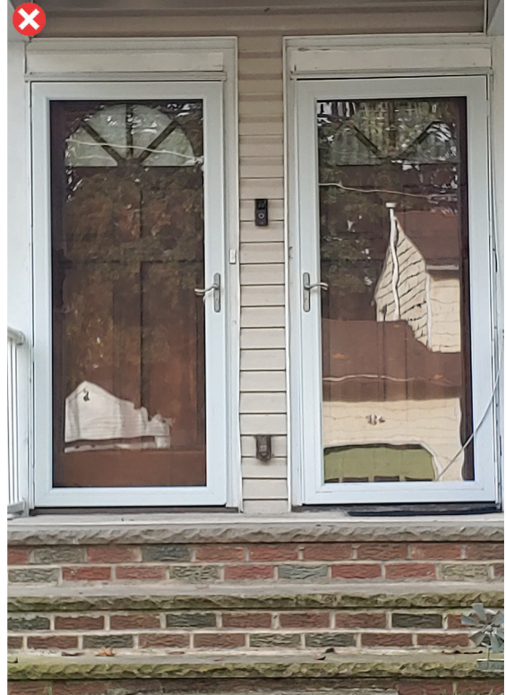
Incompatible storm door design
