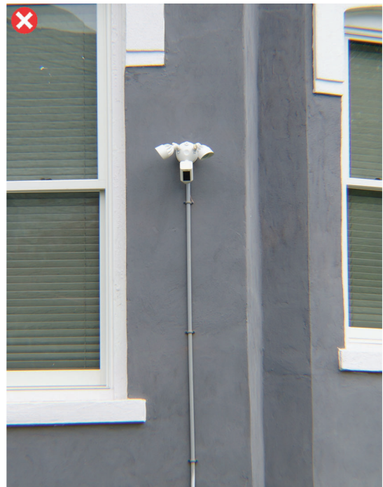
LED floodlights installed conspicuously
