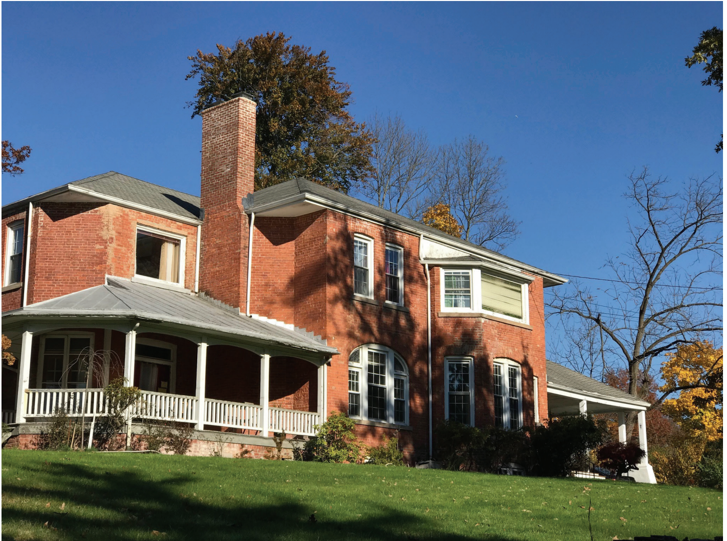
Rockview Terrace residence showing common masonry conditions on such as wearing of mortar joints and brick faces, and efflorescence (white deposits from salt in mortar)
