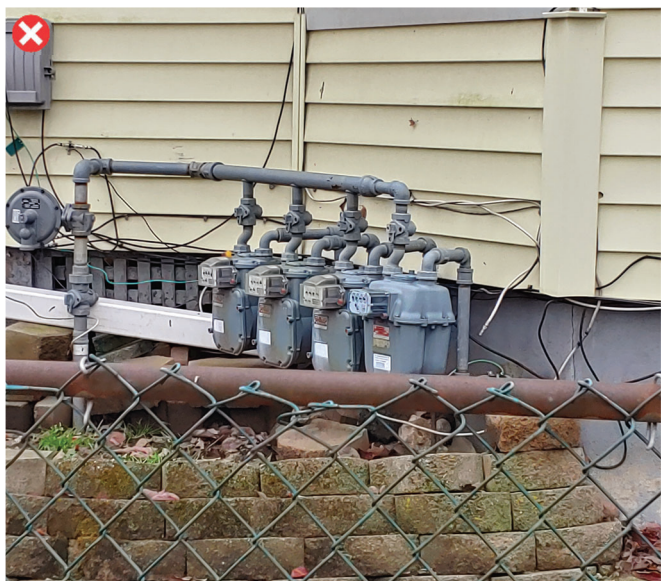
Exposed gas utility
