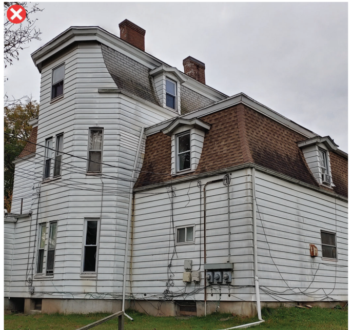
Structure is covered in vinyl siding - the impermeability of vinyl can cause condensation and degrade historic substrate
