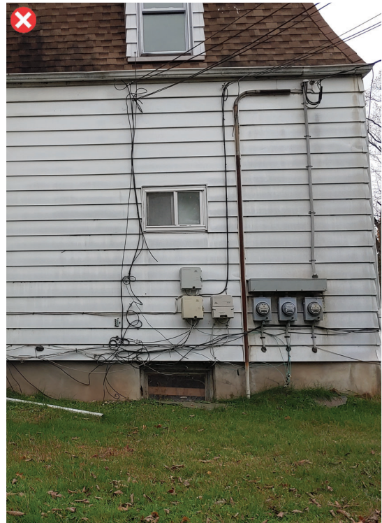
Wires not concealed
