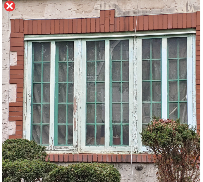
Poorly maintained wood casement windows
