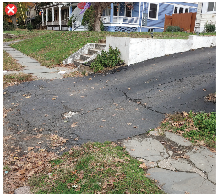
Poured asphalt in disrepair, poorly maintained flagstone walkway
