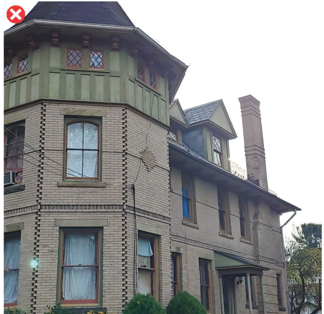
Wires attached to front elevation brickwork.
