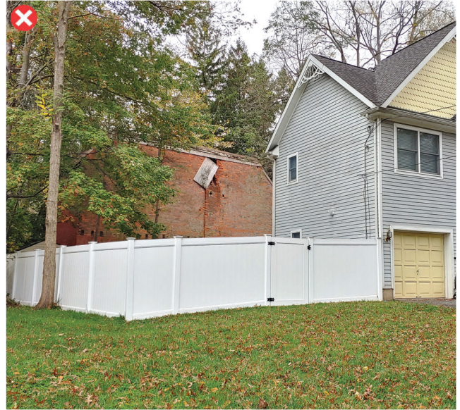
Incompatible vinyl privacy fence
