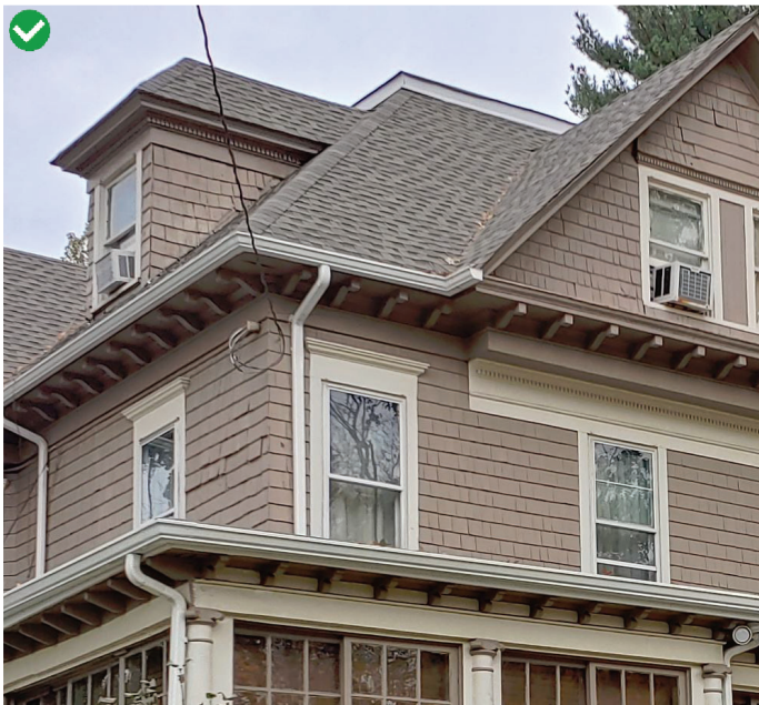
Wires attached under eaves and concealed.
