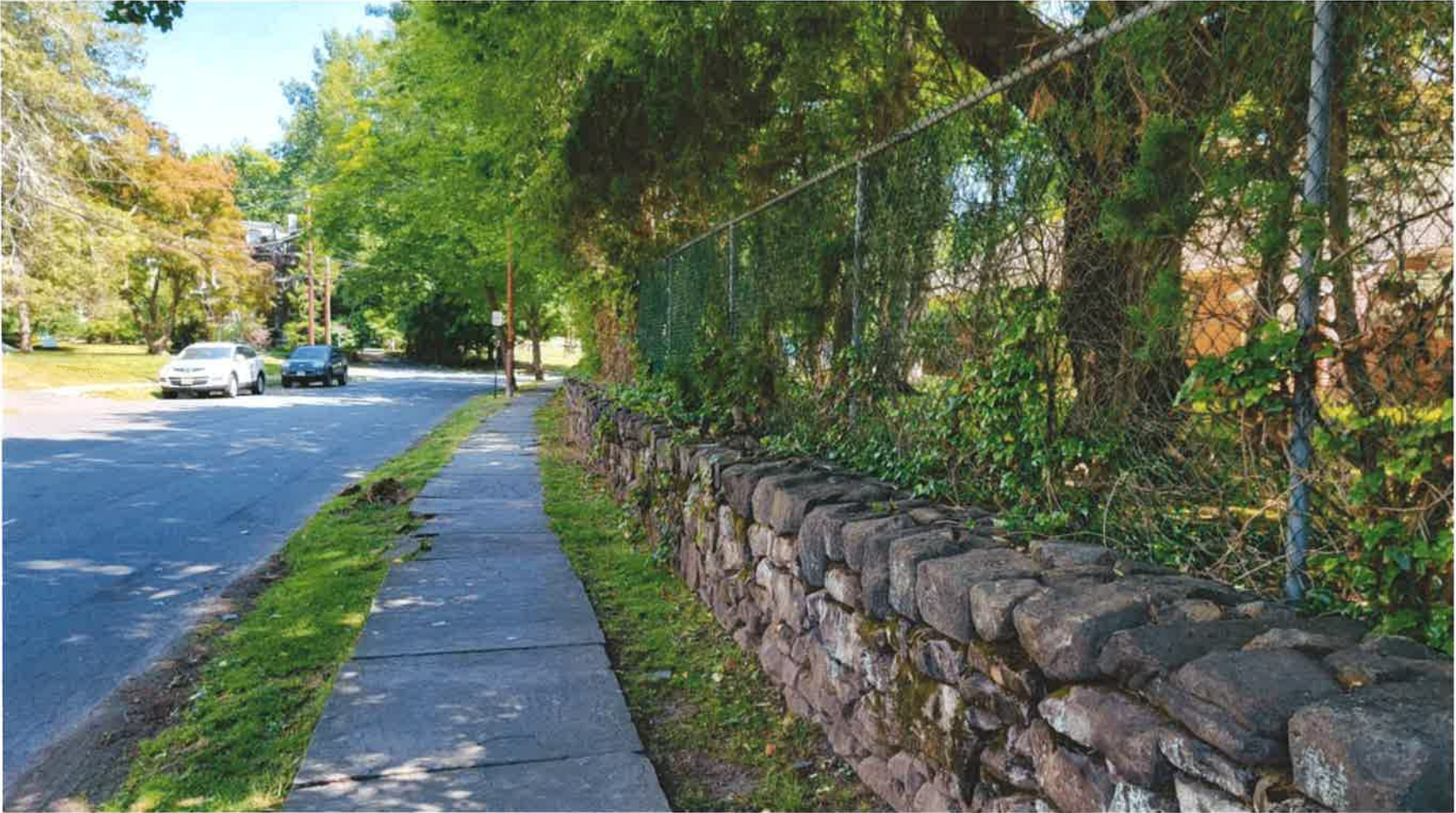
GROUND VIEW OF EXISTING PERIMTER FENCE TO BE REPLACED WITH DECORATIVE FENCE (TAKEN BY JOHN MCDONOUGH ASSOCIATES ON MAY 31, 2023)
